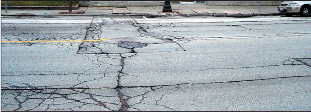
Deteriorated roadway conditions along west Central Street.
