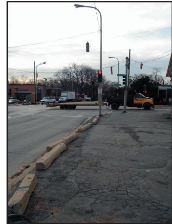
Deteriorated parking lot at CVS pharmacy.
