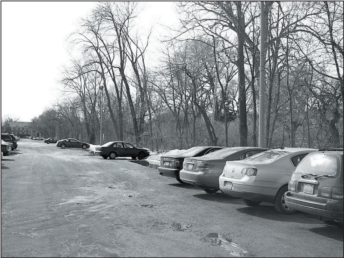
Deteriorated paving conditions and pooling water on the Ryan Field parking lot.
