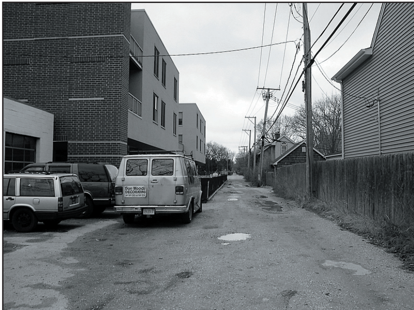
Some blocks have narrow, deteriorated and/or obstructed alleys.
