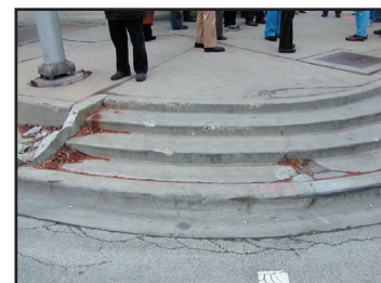
Crosswalk condition at Green Bay and Central.
