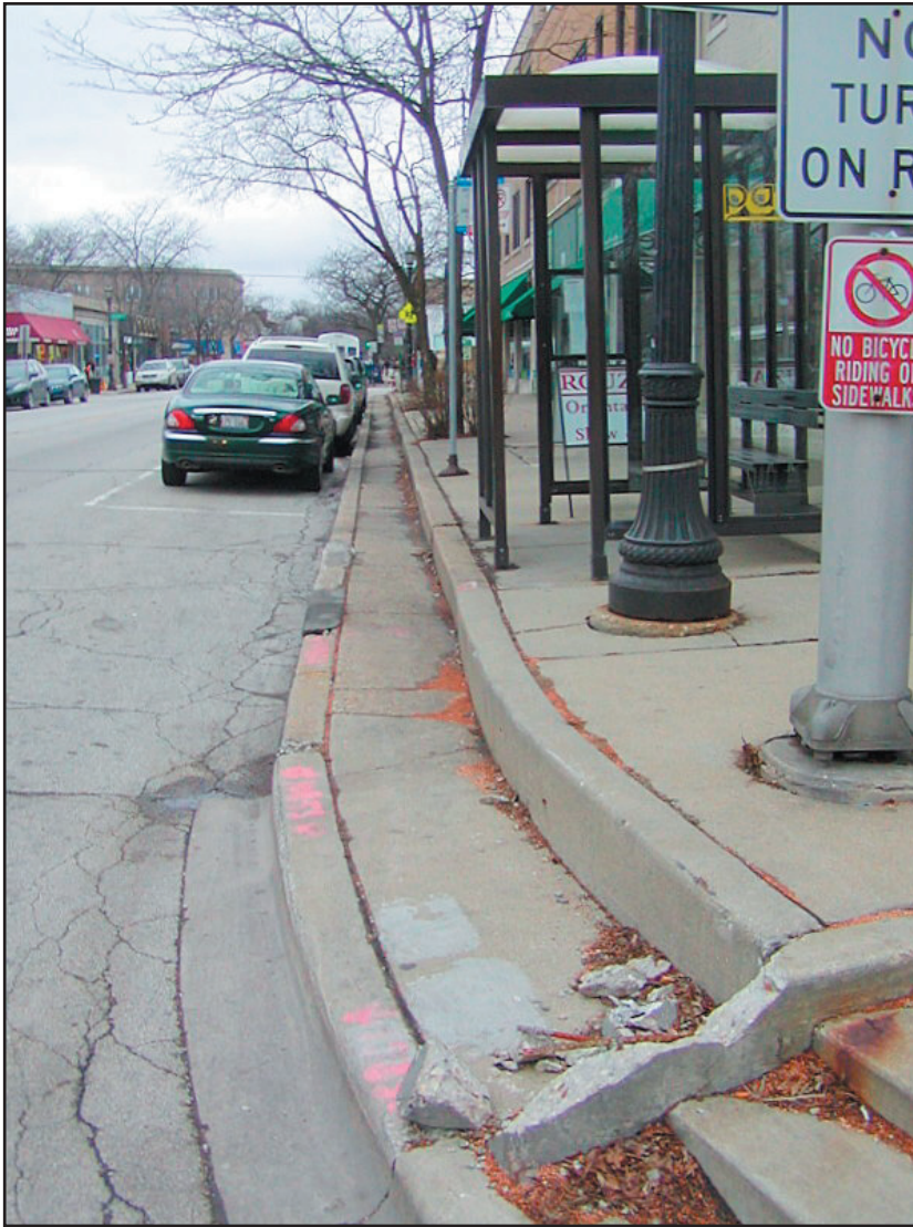
A stepped and broken curb at the intersection of Central and Green Bay.
